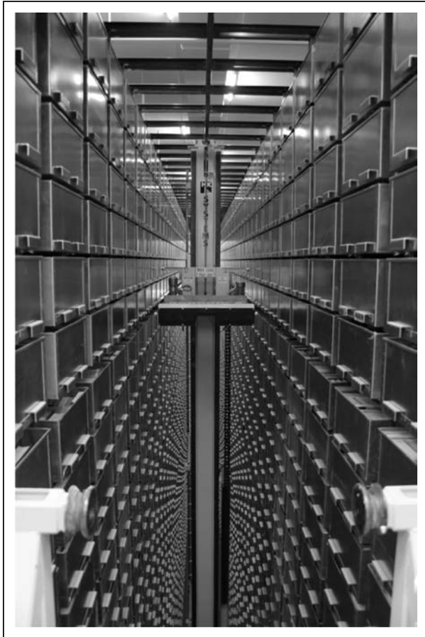
Figure 10. Automated storage and retrieval system.
